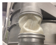
Installation gap too small
