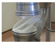
Installation gap too large
