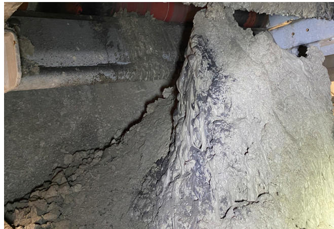
Example of incinerator bottom ash build-up under belt head drum
