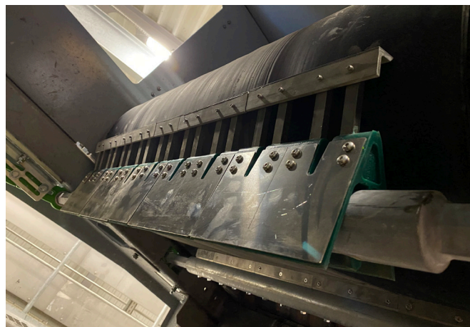
STARCLEAN® belt cleaners installed on one of the belts on site
