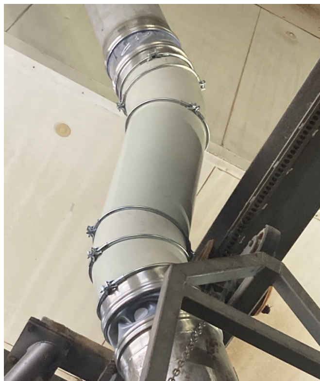
2x BFM® fittings integrated with modular pipework system
