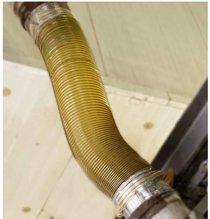
1.5m corrugated hose installed between the extruder & dryer
