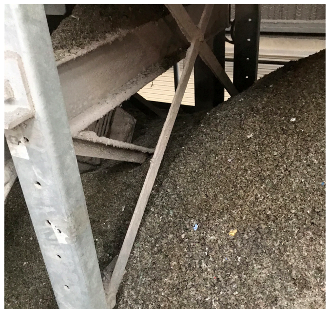
Raw material under the belt from excessive carryback
