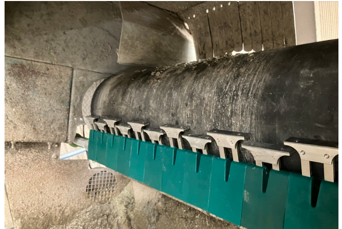
STARCLEAN® primary cleaner on the main feed belt conveyor
