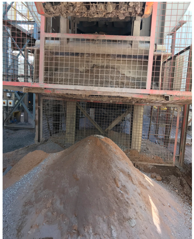
Carryback under the belt, requiring daily clean-up
