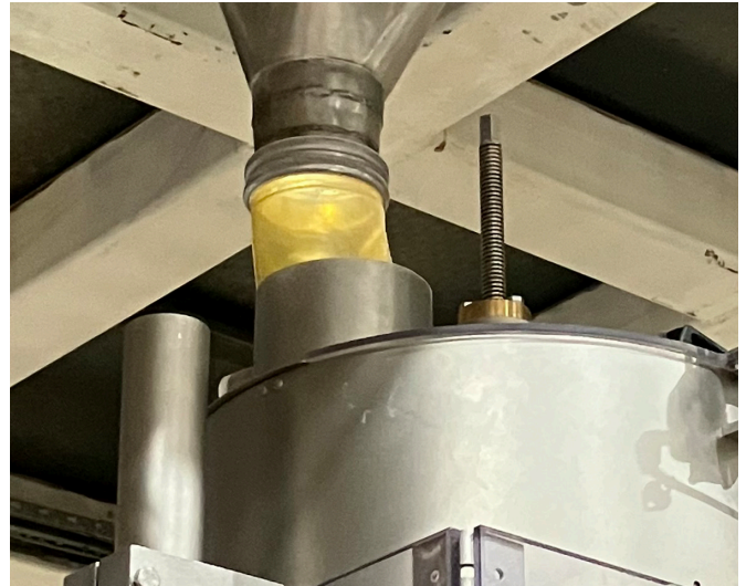
BFM® fitting installed on Richard Whittaker Ltd packing line
