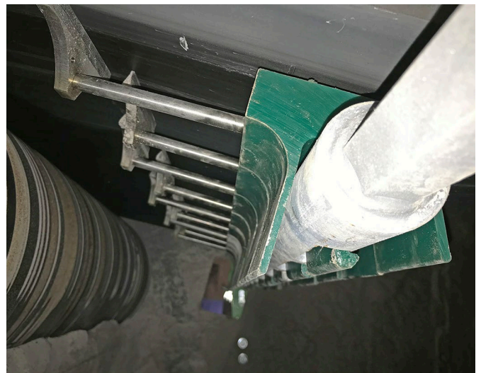
Starclean secondary cleaner in operation
